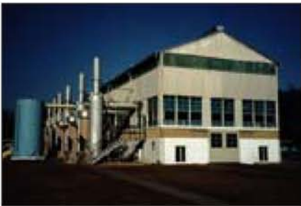
Tennessee Gas Pipeline's mainline compressor station houses five 1400 horsepower compressors.
